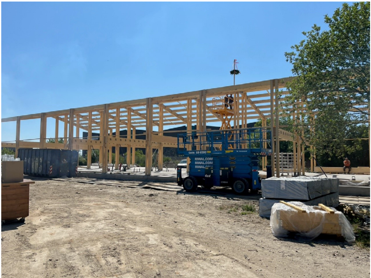
The Container Academy under construction, celebrated with a topping out event in the beginning of June, 2023.
